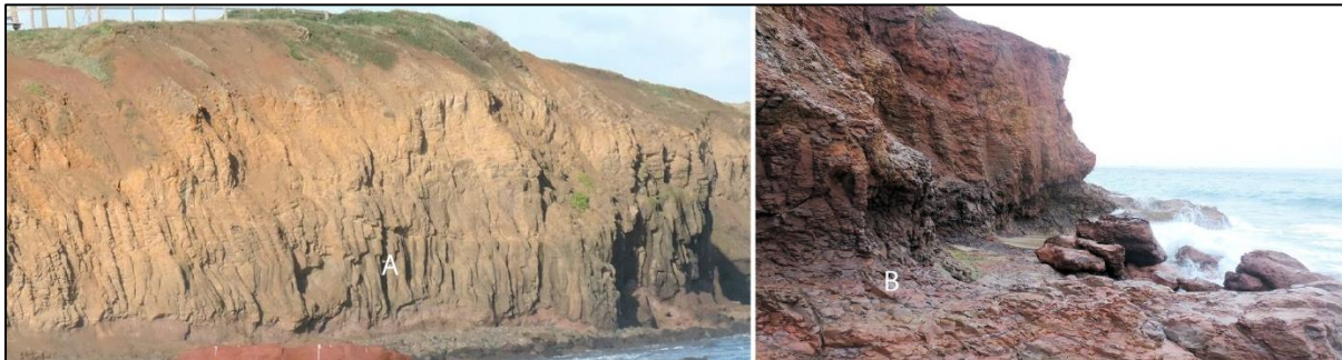
Figure 2-1 Vertical jointing in coherent basalt at Sunderland Bay (A) and close-spaced irregular jointing in fine-grained fragmental lava at Smith Beach (B)
