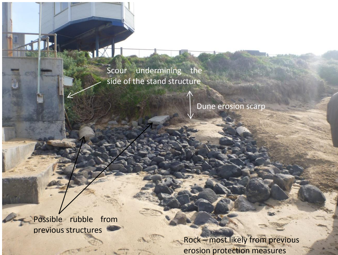
Figure 3-5 Erosion exposing and undermining sections of the concrete stands
