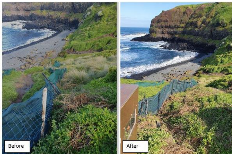
Photo - The collapsing east wing of the weighbridge pathway in Radiotracking bay; before and after repairs by Research Technical staff.
